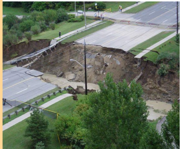
DAMAGE FROM AUGUST 19, 2005 STORM (PHOTO FROM JANE-FINCH.COM)
