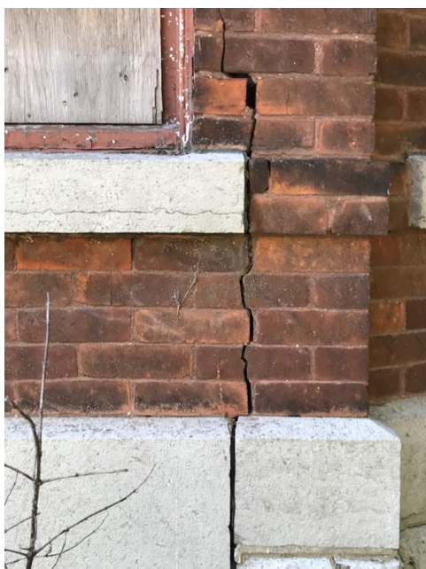
Vertical cracking, front façade
