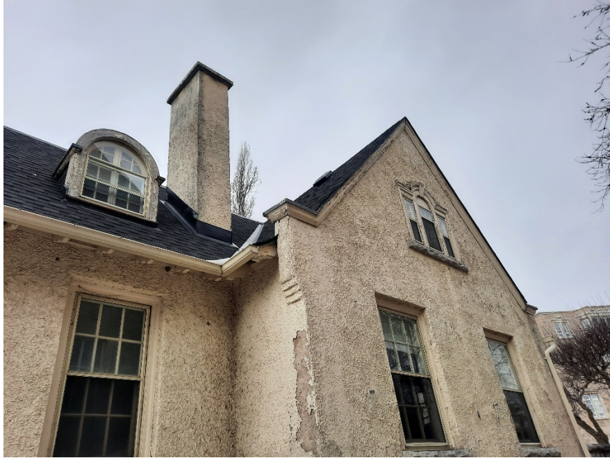
East Elevation – original wood windows, eaves, exposed rafter ends, corbelled brick courses at the base of the roof gable step
