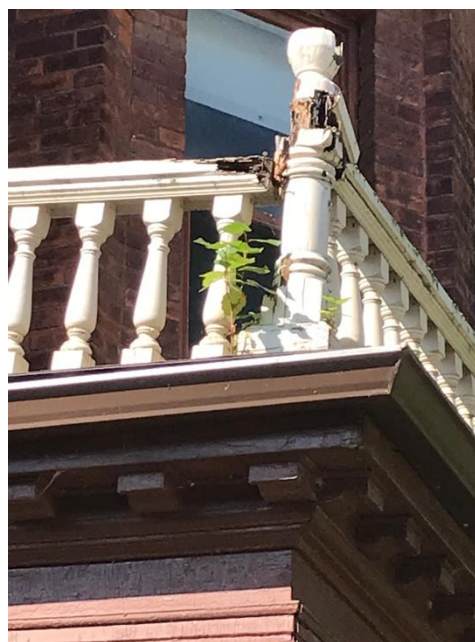
Decay of decorative wood elements, front façade
