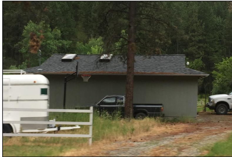
FIGURE 12 Ponderosa pine cast a considerable amount of needle litter that can accumulate on roofs and in rain gutters. The risk here is of ember ignition of the needle litter and subsequent ignition of the roof. Periodic removal is recommended to keep these hazardous fuel accumulations to a minimum.
